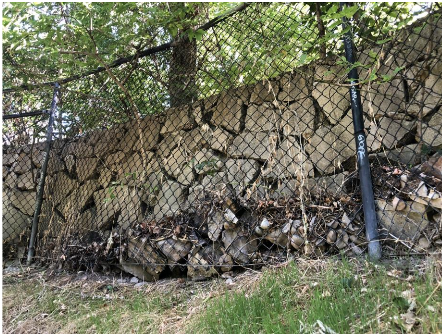
Photo #16 – There is a retaining wall built above the original rock wall that has large rocks caught in the fence. This wall is an example of neighbors building structures above the existing walls and creating additional loads on the existing structure.
