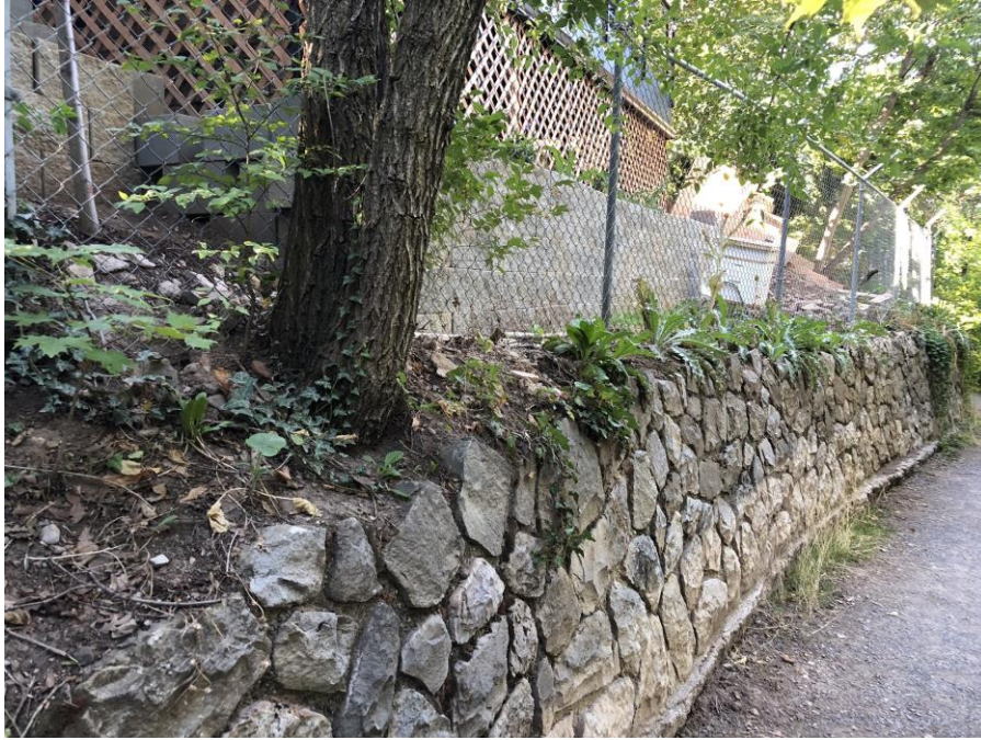
Photo #13 – Example of neighboring property owners building structures above existing rock walls. Trees that occur adjacent to the wall should be removed and the structural fill should be used to backfill over the toe of the existing rock wall.
