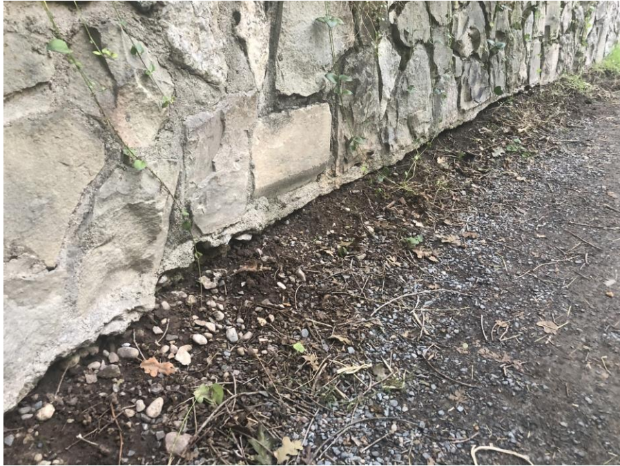
Photo #1 – Soil cover over toe of wall is not adequate
