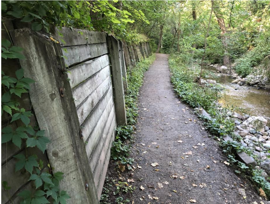
Photo #3 – Runoff from adjacent property owners' gutters is causing the wall to bulge and fail
