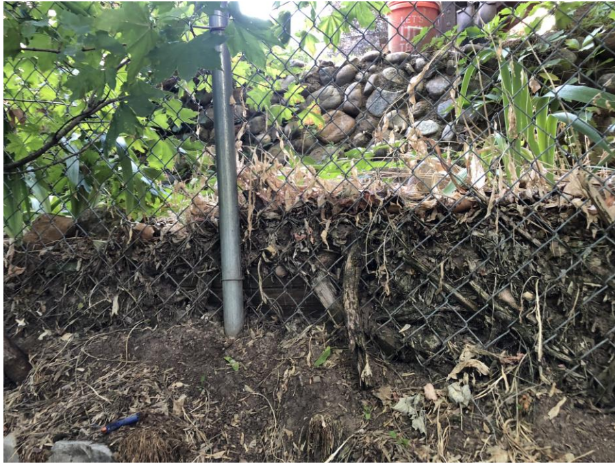
Photo #7 – Chainlink fences are collecting debris from runoff water and are retaining soil.
