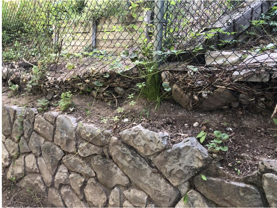
Photo #9 – Chainlink fences are collecting debris from runoff water and are retaining soil.
