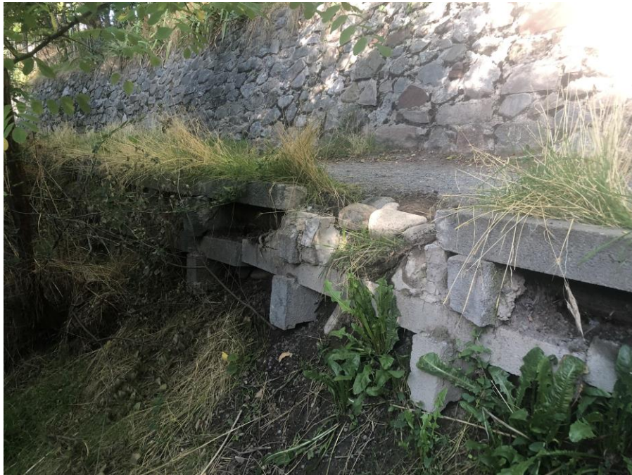
Photo #2 – erosion on the trail due to runoff and sprinklers has cause the crib walls to fail in several locations.
