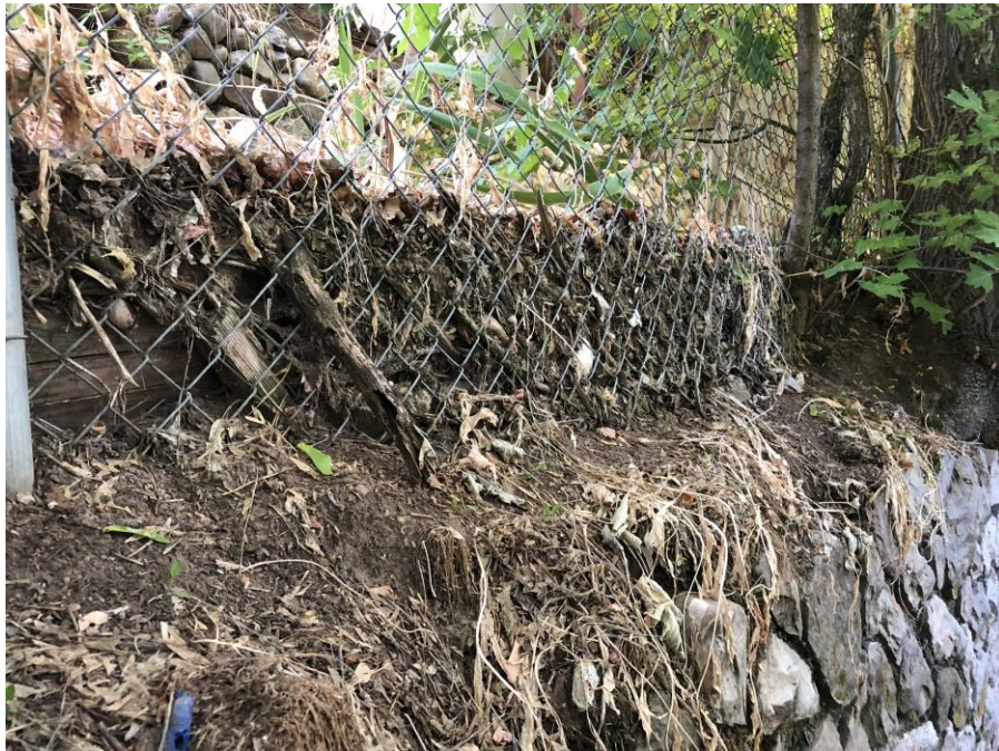
Photo #8 – Chainlink fences are collecting debris from runoff water and are retaining soil.
