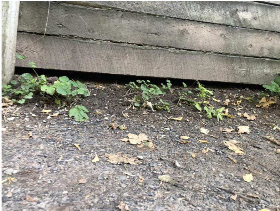
Photo #4 – Runoff from adjacent property owners is undermining existing walls.
