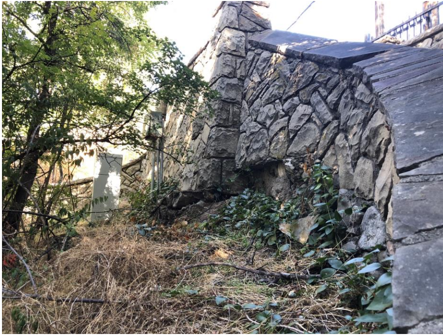
Photo #17 – The existing wall is being undermined and the toe needs to be covered with structural fill.
