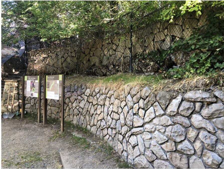
Photo #15 – There is a retaining wall built above the original rock wall that has large rocks caught in the fence. This wall is an example of neighbors building structures above the existing walls and creating additional loads on the existing structure.
