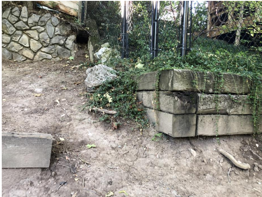
Photo #10 – Image of drainage from neighboring property owners and runoff from sprinklers causing the soil to erode and undermine the existing retaining wall structures.
